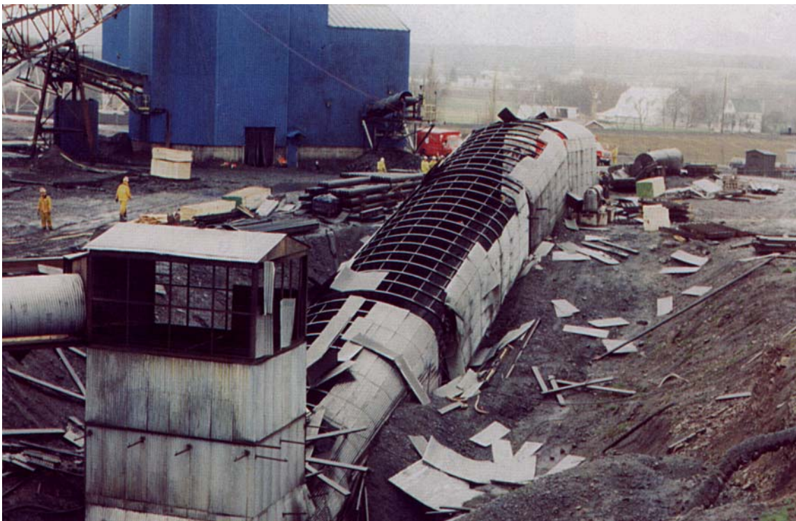
Figure 3 Damage to portal at No. 1 main, Westray coal mine (from Richard, 1997).
